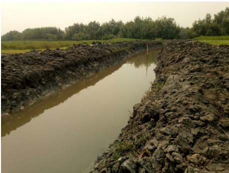
The central canal that was built to let in water to the restoration site at Djébadji, Ouidah, Benin.
